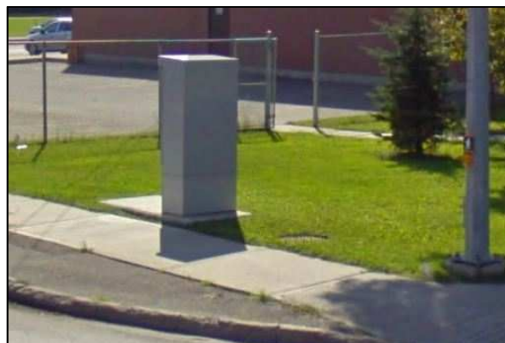
2 Typical Traffic Signal Switchbox
