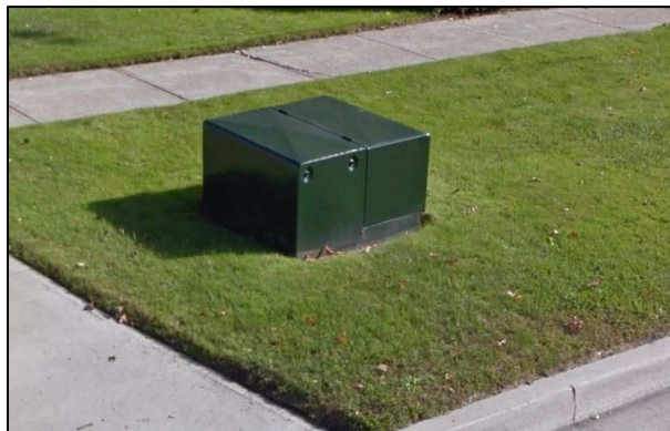
3 Typical Surface Hydro Vault
