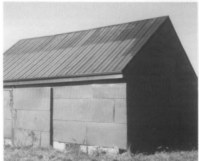
Figure 9. Severely deteriorated wooden siding on a farm building has been covered over with painted plywood panels as a temporary measure to eliminate moisture penetration to the interior. Foundation vents and loose floor boards allow air to circulate inside.
