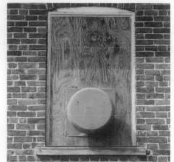
c. The exhaust fan has tamper-proof housing.
