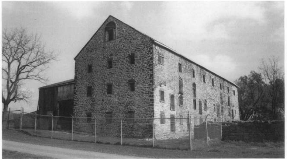
Figure 24. Once mothballed, a property must still be monitored and maintained. The openings in this historic barn has been modified with a combination of wood louvers and metal mesh panels which require little maintenance. The grounds are regularly mowed, even inside the chain link security fence. Photo: Williamsport Preservation Training Center, NPS.
