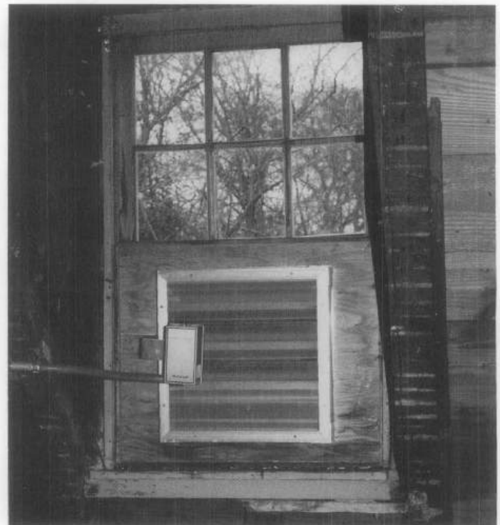
Figure 21. This electric thermostat/humidistat mounted in the attic vent controls a modified ducted air/fan system. The unit uses temporary exposed sheet metal ducts to pull air through the building and exhaust it out of the basement. For over ten years this fan system in combination with 18" x 18" preformed louvers in selective windows has kept the interior dry and with good air exchanges.
