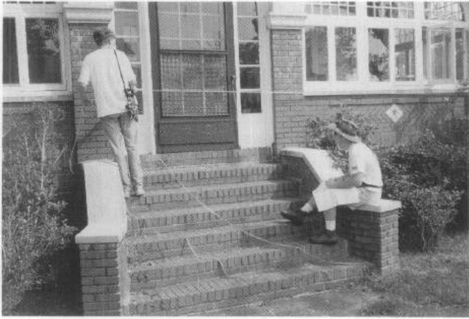
Figure 4. Documenting the building's history, preparing schematic plans, and assessing the condition of the building will provide necessary information on which to set priorities for stabilization and repair prior to securing the building. Photo: Frederick Lindstrom, HABS.
