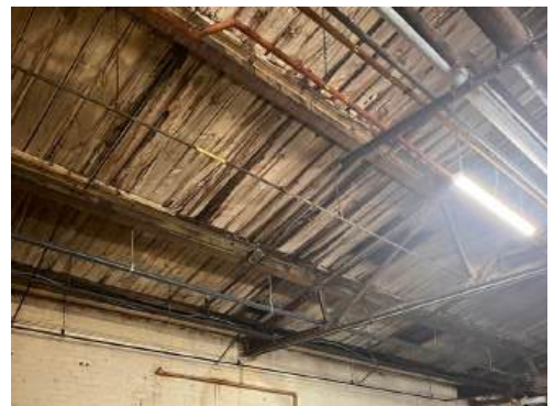
32. Interior water damage to ceiling (ERA, 2023)
