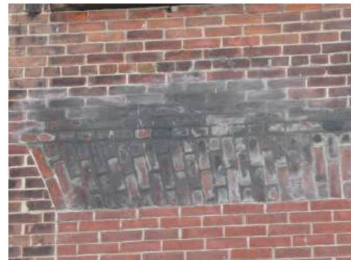
28. Masonry staining and efflorescence (ERA, 2023)
