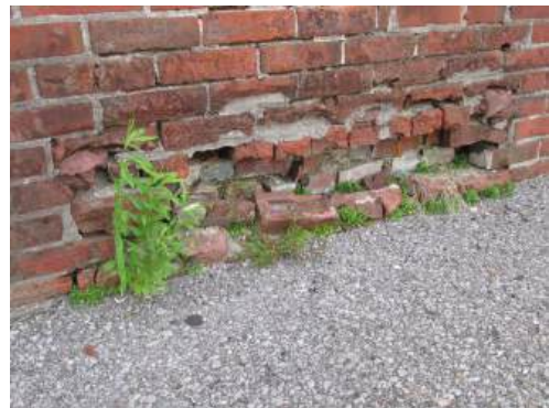
24. Brick deterioration and unsympathetic repair(ERA, 2023)
