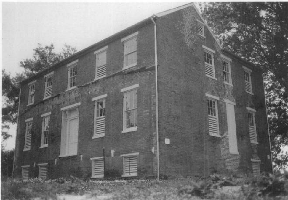
Figure 1. Proper mothballing treatment: This building has been successfully mothballed for 10 years because the roof and walls were repaired and structurally stabilized, ventilation louvers were added, and the property is maintained. Photo: Charles E. Fisher, NPS.
