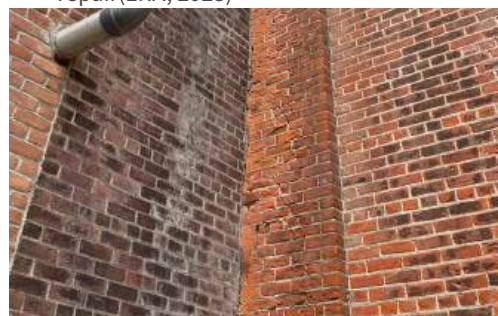
25. Brick deterioration at intersection of buildings ERA, 2023)
