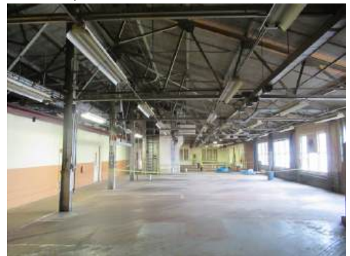
33. Area of roof leak damage, Building 30 (ERA, 2023)
