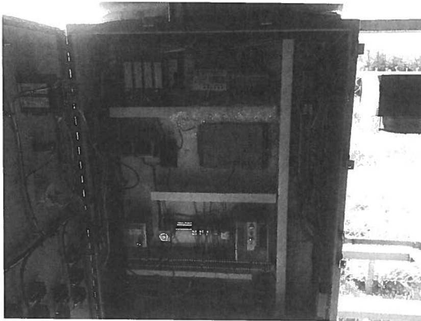
System Control Panel
