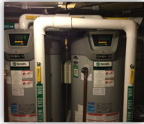
Hot Water Tanks 53 Spring Street Norwood
