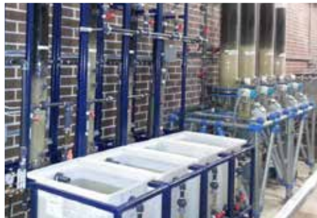
Above: Biofilters added at the Peterborough WTP Pilot Plant
